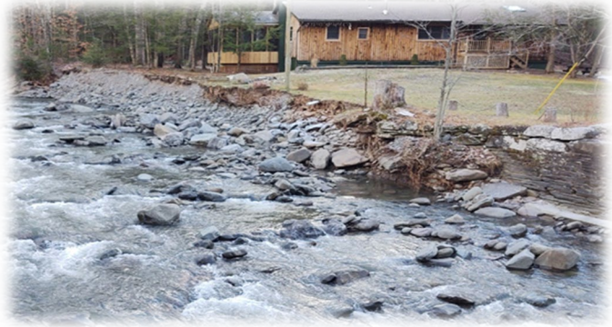
Rock Armoring 1 year after installation near Woodstock, NY. Note further failure and bank alignment has retreated nearly 20 feet toward home. Future UCSWCD riparian buffer project site.
