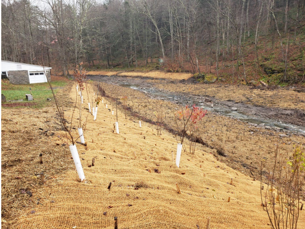
Figure 2: Post-construction showing remediated terrace and planform and hydraulic geometry adjustments with native plantings.
