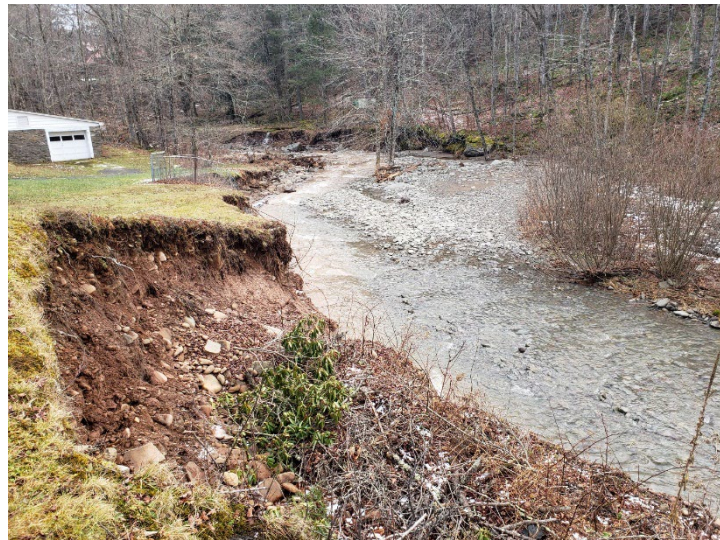
Figure 1: Pre-construction showing eroding terrace and suspended sediment generation from exposed glacial sediment.
