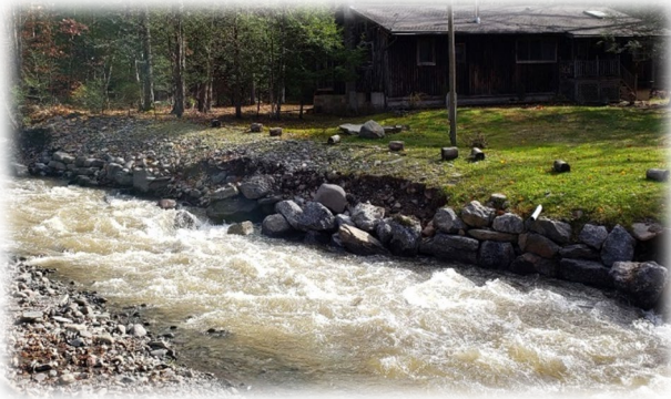
Rock Armoring along turf lawn 1 month after installation near Woodstock, NY. Note rocks already falling into stream channel after being undercut by floodwater.
